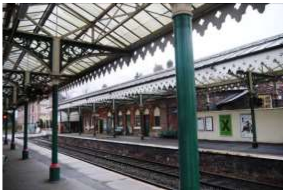
Detail of the decorative elements within Character Zone B including iron capitals, pierced timber valance and polychromatic brickwork
