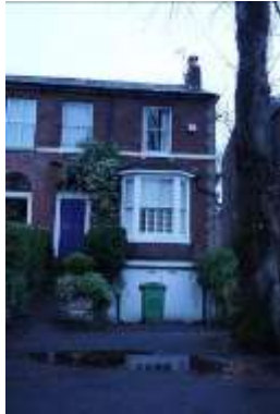
Inappropriate converted basement garage at 12 Spring Road
