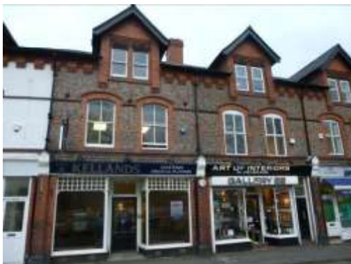
Historic shop fronts along Victoria Road with slim timber glazing bars and recessed doorways (Character Zone A). The glazing bars to the right were removed in 2015, which is harmful to significance.
