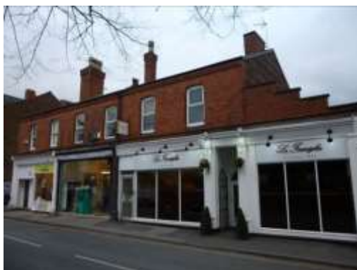
Inappropriate shop front with no stall riser and a large expanse of glass with no glazing bars at 16 Victoria Road (Dress 2 Party). The darkened glazing at 12-14 is also not appropriate.
